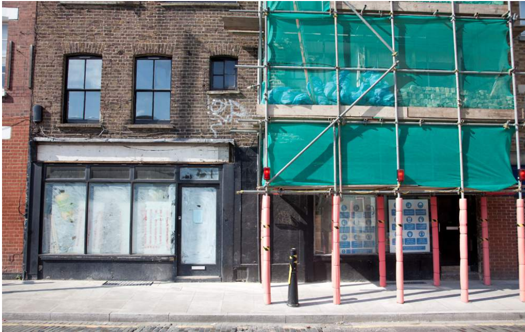
The condition of existing elevation which will be reinvigorated to improve the street scene as a result of the proposals.
